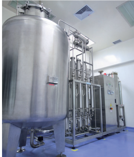
Flow measurement of demineralized water
